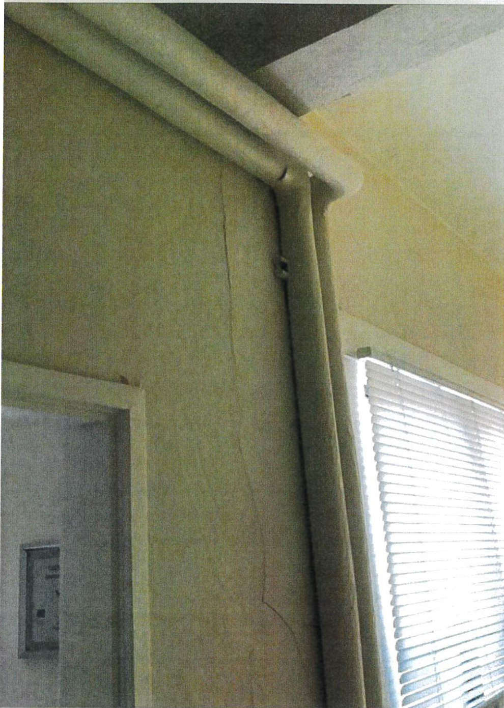
Photo 1 – Crack Below Beam at Room C2
